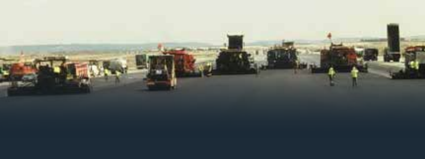
Echelon paving the main runway on the Charles De Gaulle airport in Paris.
